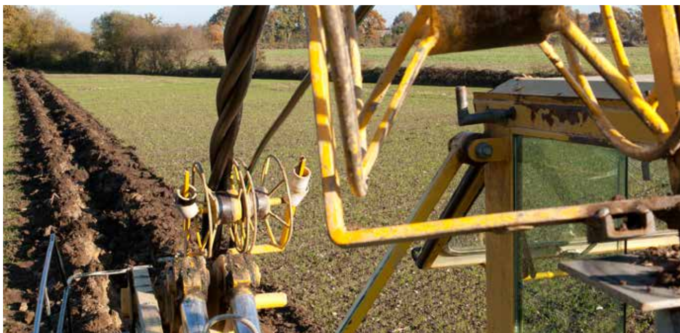
Example of mechanized installation: 3 pre-assembled single cores laid at the same time and directly buried.
